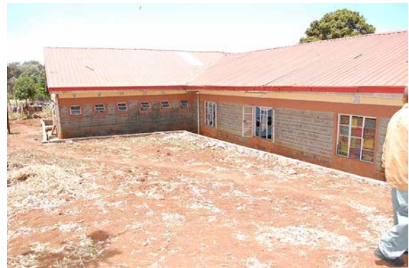
Protective trough at base of Boys' Dormitory
